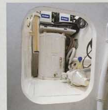
Dedicated pump room
